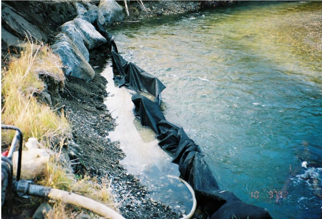
Figure 3. Photo of a method to isolate the stream edge to allow for the installation of armoring or rip rap. A pump is used to contain/remove dirty water from the enclosure.
