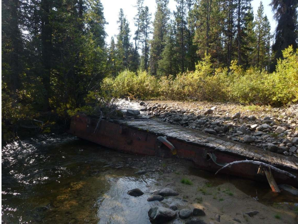
Photo 27. The washed-out bridge 50 m downstream of the crossing and partially buried by fluvial material.
