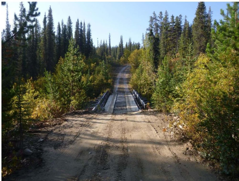
Photo 8. View of the bridge at Site 2 looking south. Note the slight slumping of the north side of the bridge on the left side of the photo.
