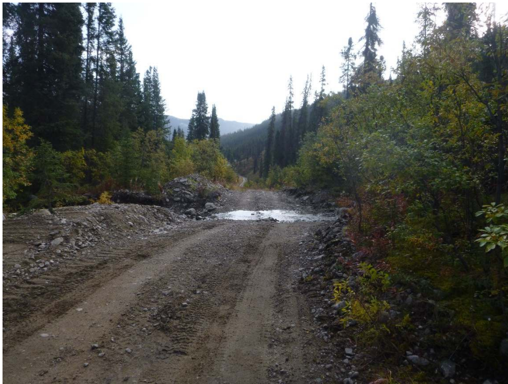
Photo 28. View of the ford crossing at Site 10, with the creek flowing over the road.
