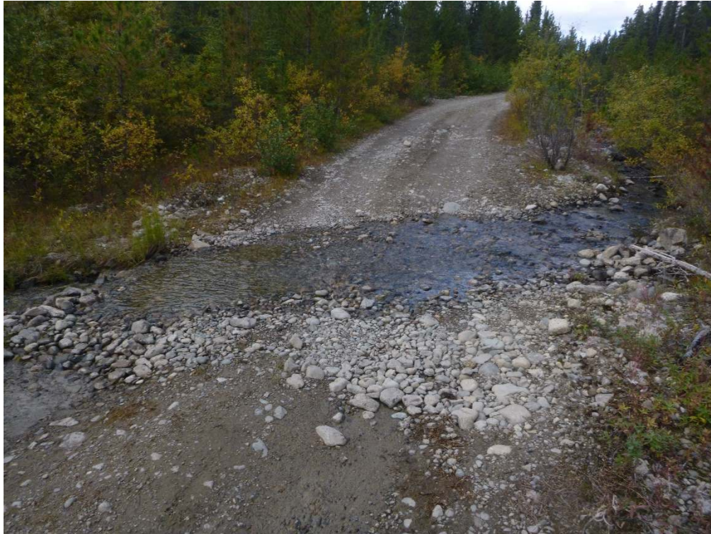
Photo 10. Water flowing over the access road at Site 2B.
