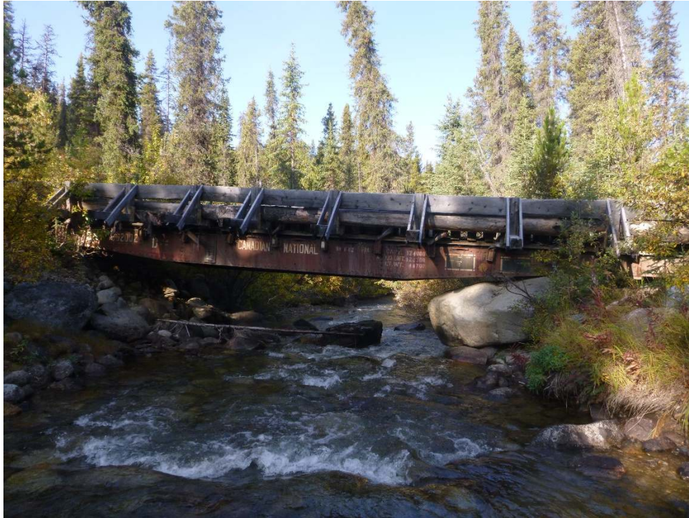
Photo 7. Downstream view of the bridge at the Site 2 crossing from Goat Creek.
